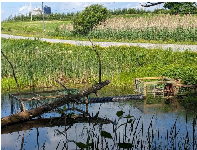
Beaver Deceiver™ Device installed at a culvert in Charlotte
